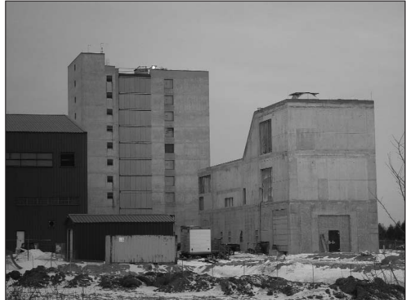
Construction of full-scale fire research facilities adjacent to existing NRC facilities at Almonte, Ontario is underway.
