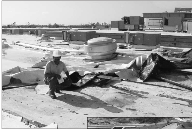
Dr. Bas Baskaran points out the extensive roof damage as the result of a hurricane.
