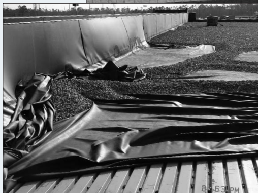
Ballasted roof is completely blown off by wind (top and middle).
