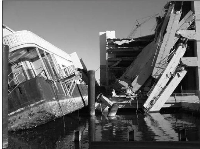
Post-tensioned parking garage severely damaged by a casino barge moored alongside
