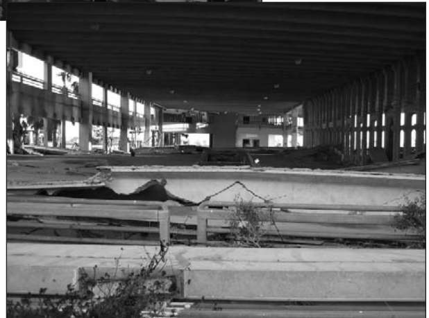
Collapsed precast parking garage deck, apparently caused by the lateral and uplift forces of the storm surge
