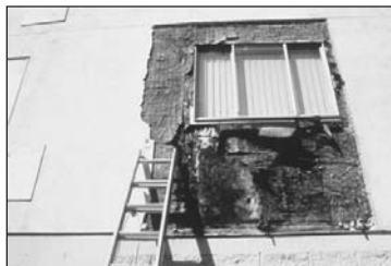
Premature deterioration of sheathing board and wood studs adjacent to a flanged window.
