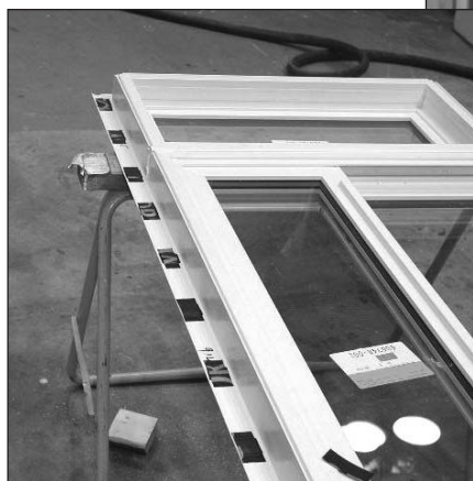
Mounting flanged window on furring strips (above), or using shims behind the flange (left), provides the openings necessary for proper drainage.
