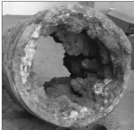
Drinking water may contribute to the deterioration of pipe materials.
