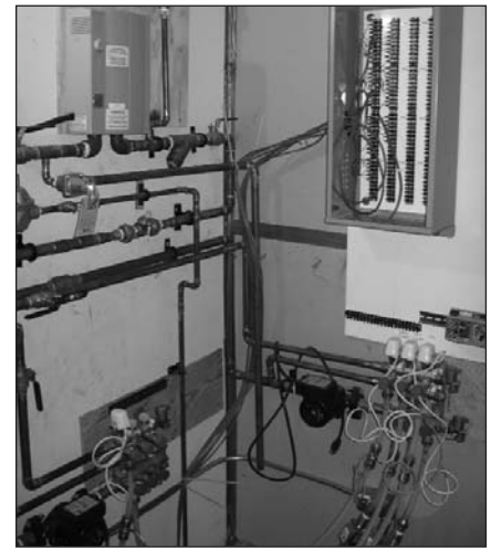
Boiler system for Ventilation and Wall Research House
