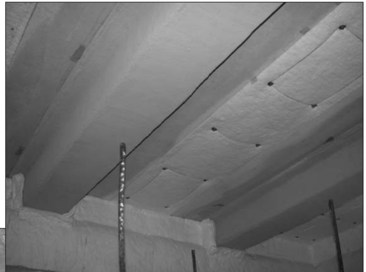
a) Before fire test
