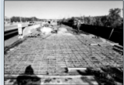
The rehabilitation of deteriorated bridge decks accounts for one third to one half of bridge maintenance costs in North America.
