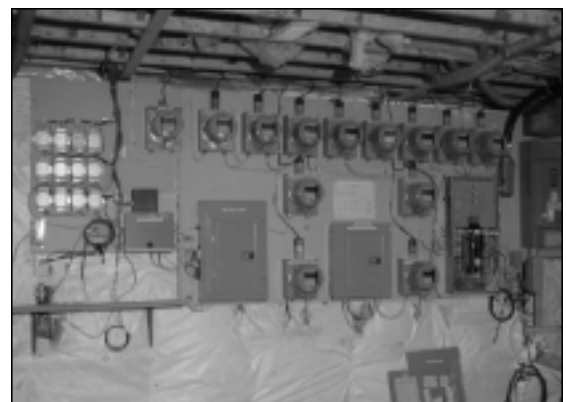
New meters at CCHT are able to characterize the electrical consumption of the houses for each five minutes of a 24-hour period.
