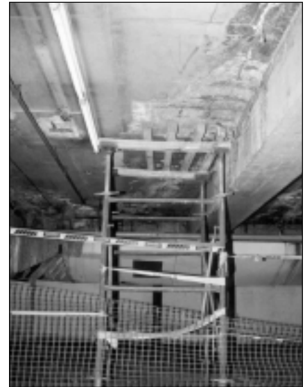
Typical deterioration found in parking garages
