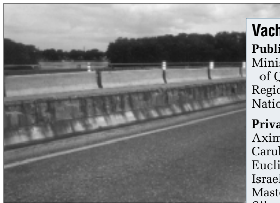
Vachon Bridge parapet wall shows significant corrosion prior to installation of corrosion inhibiting system.
