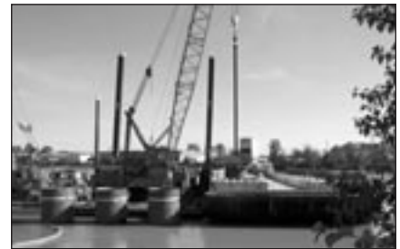
Innovative caisson dredging technique by Fraser River Pile and Dredge Ltd. wins CCA Excellence in Innovation Award.
