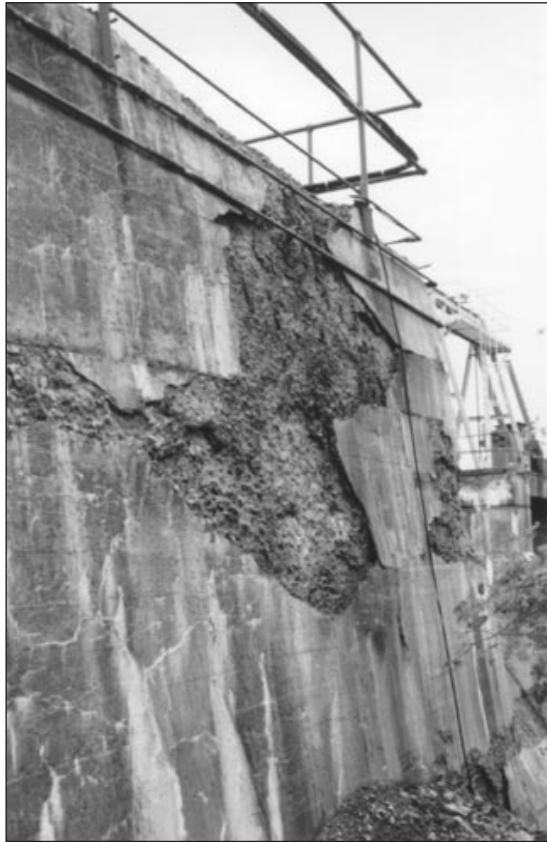
Figure 2. Example of freeze/thaw damage
