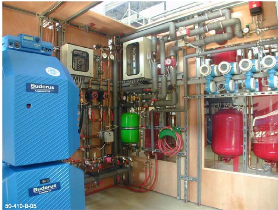
Figure III-1.1 : Test rig for heat generation
