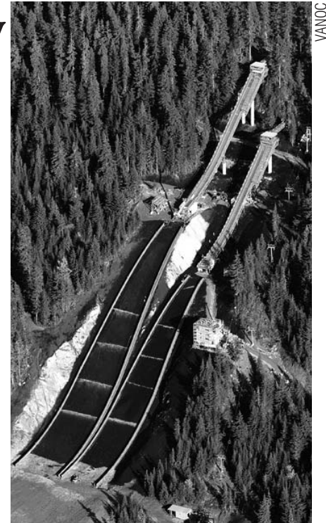
The Whistler Nordic Centre ski jump area is just one of the new venues under construction for the Vancouver 2010 Winter Olympic Games.
