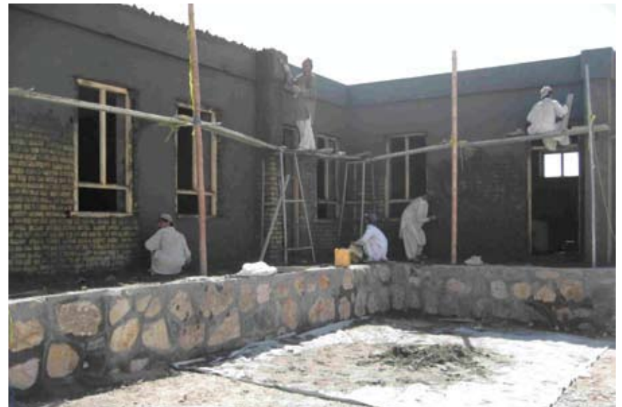
Through Canada's education signature project, Canada is investing up to $12 million over three years to build, expand and repair 50 schools in targeted districts in Kandahar province. Photo: One of the Canadian schools being built in Afghanistan.
