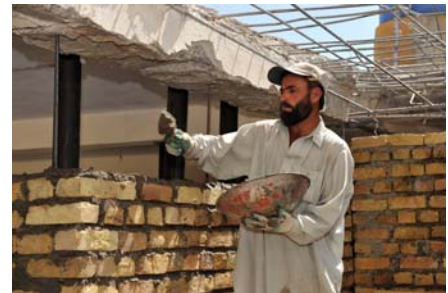
A local Afghan repairs a building of the District Centre in Deh-e-Bagh, Kandahar province.
