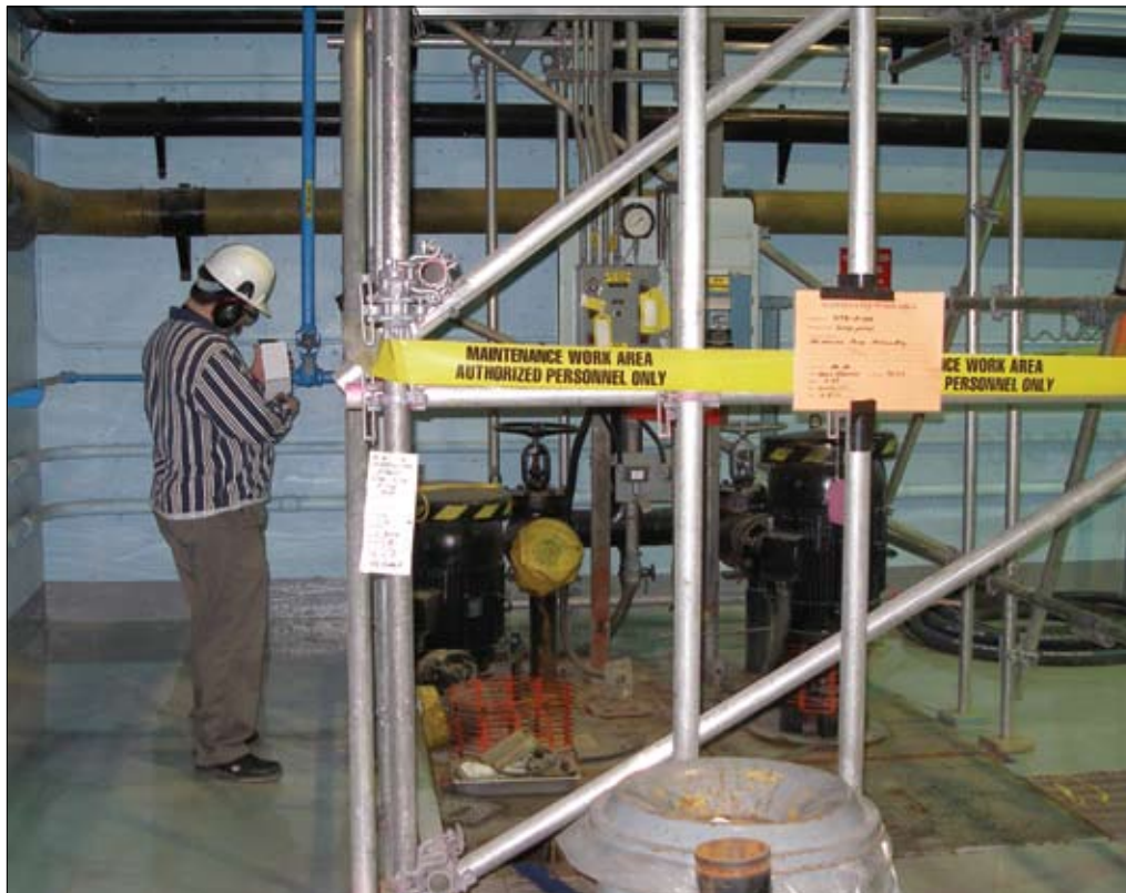
CHECKING TURBINE SUMP PUMP LEVELS TO ENSURE THEY ARE WORKING EFFECTIVELY.
