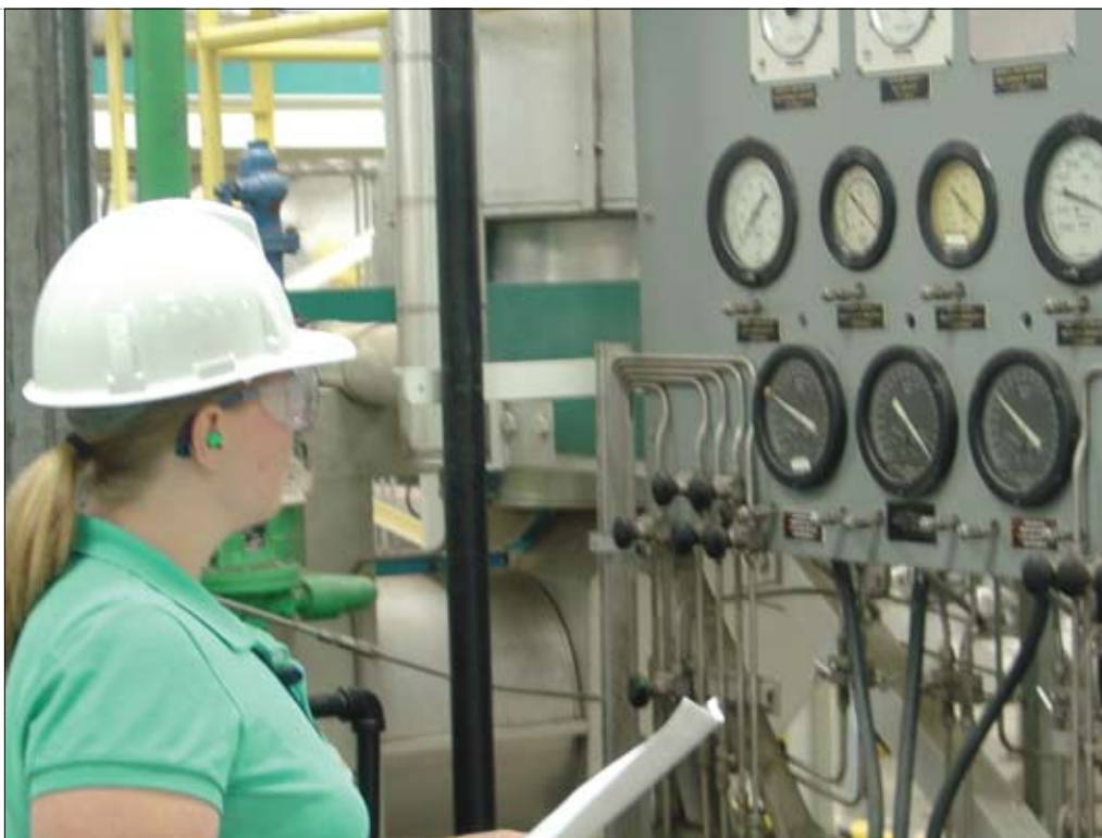
CHECKING GAUGES TO ENSURE ADEQUATE PRESSURE OF THE BOILER FEED PUMP.
