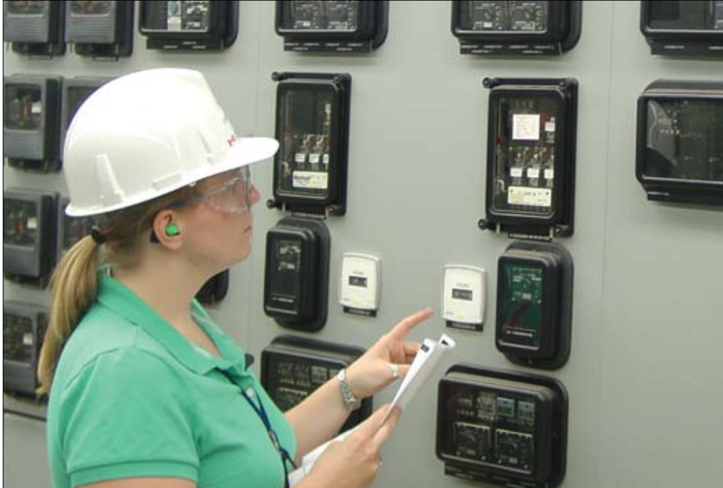
CHECKING THE RELAY PANEL.
