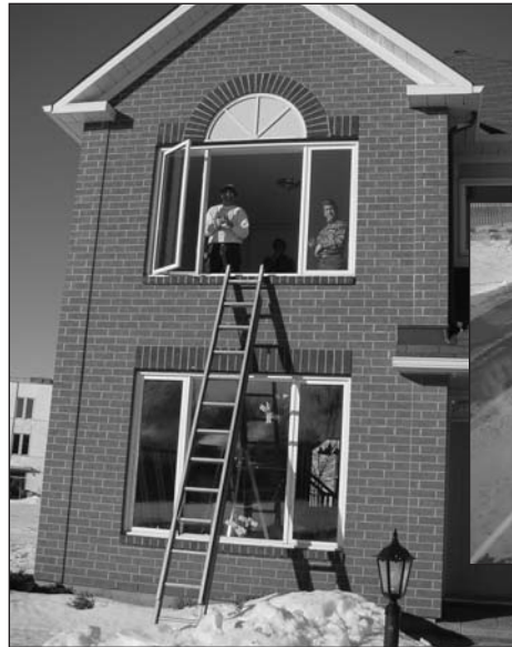
Changing the windows in the CCHT Test House in preparation for the experiment
