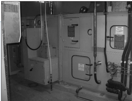
The facility's air handling system
