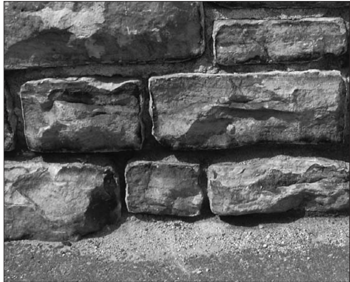
Figure 3. Damage from frost and salt results in erosion of the mortar.
