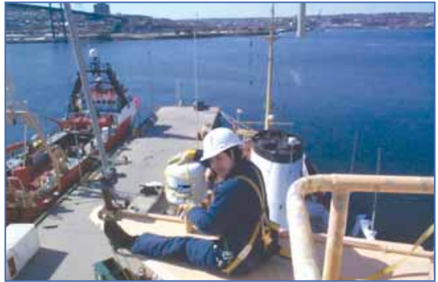
Electronic maintenance technologist Mylène DiPenta replacing a satellite antenna at the top of the main mast on CCGS Hudson , Offshore Oceanographic Science Vessel
