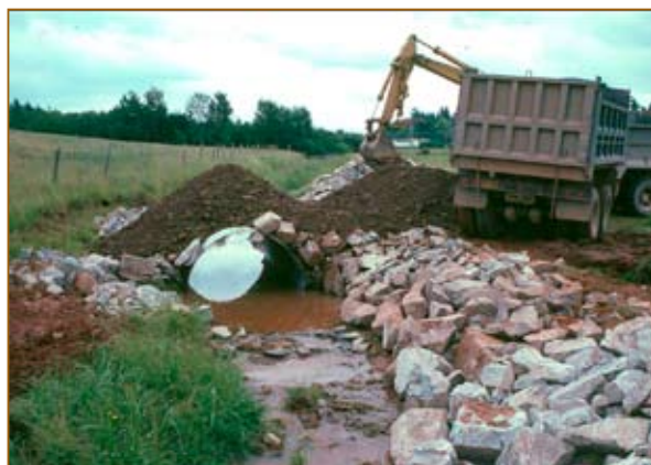
Installation of the culvert crossing and stream bank-stabilizing rip-rap. Photo: Ken Webb.
