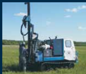
Drilling rig for seismic shot holes at Big Island Lake Cree Territory, Saskatchewan.
