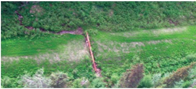
FIGURE 44. This reclaimed site is well contoured and revegetated, but the culvert should be removed.
