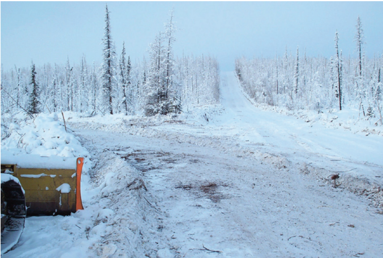
FIGURE 8. Verifying the route prior to construction can avoid unnecessary false starts such as this one
