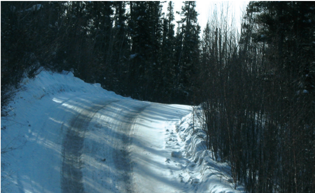
FIGURE 6. Road grades and curves should be designed to be safe and minimize environmental disturbance. In this case, a wider curve and a lower grade would be safer and less prone to erosion.
