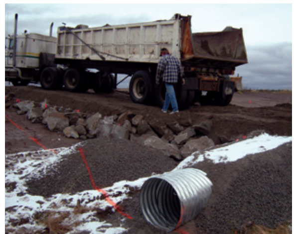
FIGURE 17. This cross drain is covered with coarse-grained granular material for frost protection.
