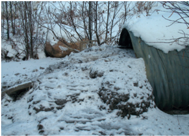
FIGURE 38. Culverts should be monitored and cleaned regularly to ensure that they continue to function properly.
