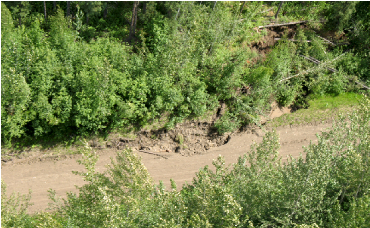
FIGURE 37. Regular monitoring will identify areas prone to erosion that may need to be redesigned.
