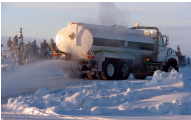
FIGURE 30. The road surface can be built up with ice using a water truck with a sprayer.
