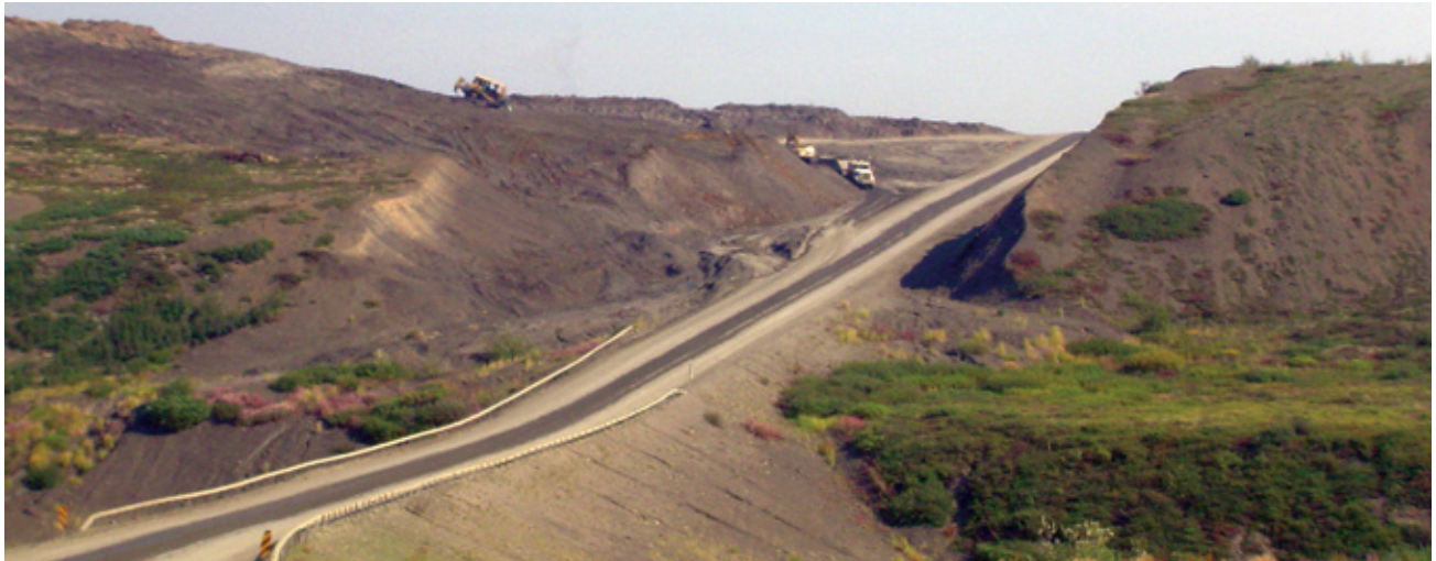
FIGURE 16. The slope of this road has been reduced by fill excavated from the adjacent cut. Drainage and Erosion Controls
