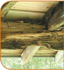
Carpenter ant damage on porch roof Photo: Gerry Duprey
