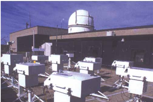
Brewer spectrophotometers located on top of the Environment Canada building in Toronto.
