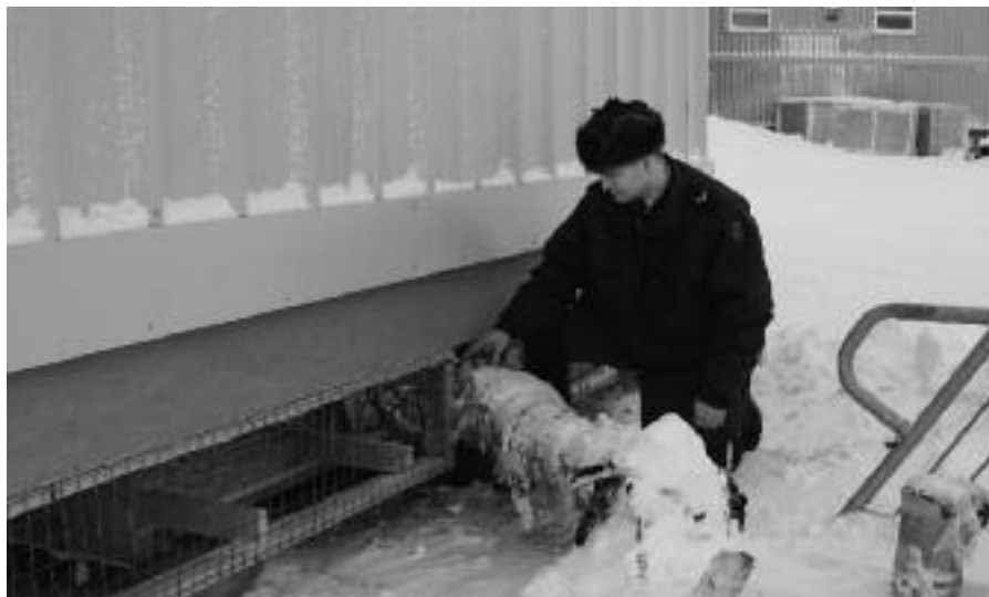
Cpl Doug Schiffner, serving on relief in Coral Harbour, Nunavut, examines repairs that he, Cpl Shaun Haubrick and a local resident made to the detachment sewer pipe after it burst. The trio used plastic, duct tape and a good dose of ingenuity to complete their work.
