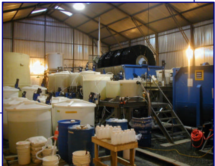
Two pilot water treatment plants at Colomac Mine, NWT
