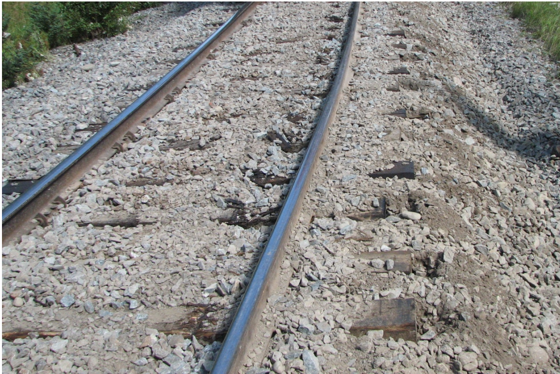
Photo 1. Disturbed ballast at ends of ties
