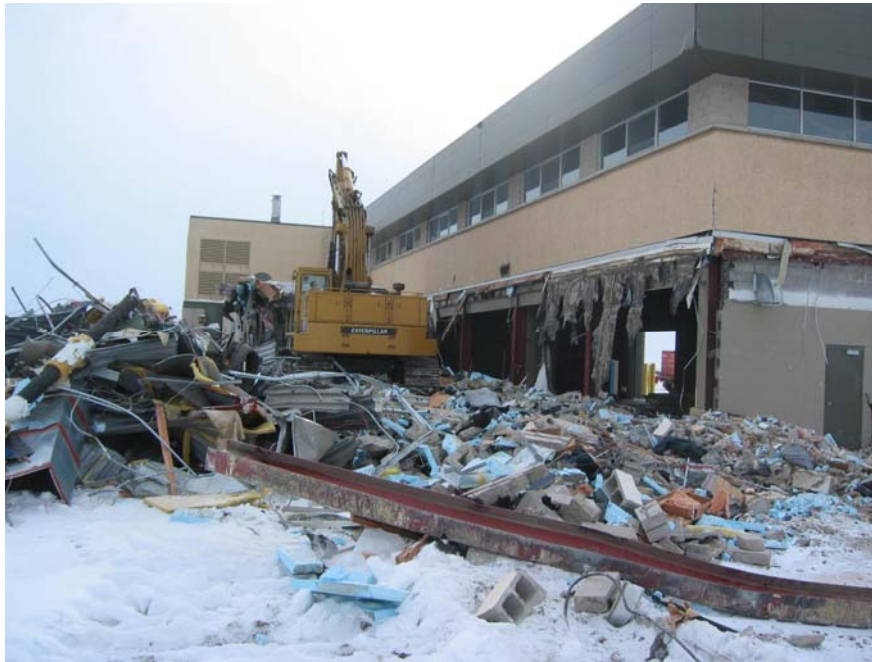
DCC coordinated the demolition and removal of the German Army Training Establishment Shilo (GATES). Room has been cleared for more modern developments for this Area Support Unit, as well as the increased influx of troops through the addition of the 2 PPCLI Regiment.
