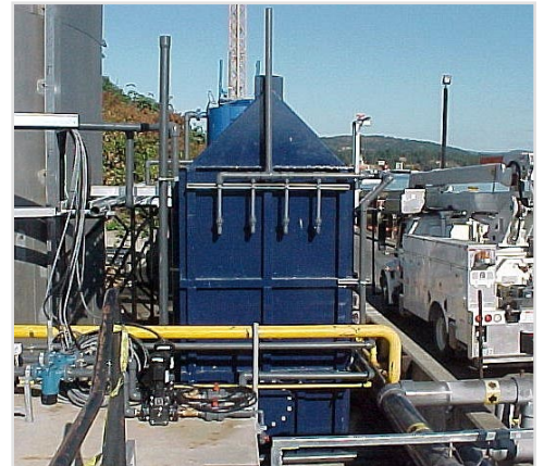
The Floc Separator, also known as the "Volcano," separates the coagulated molecules from the water. The water then enters the sand filters, while the floc, or sludge, is pumped to the pressure filters. This intricate piece of machinery is part of CFB Esquimalt's new oily wastewater treatment plant.
