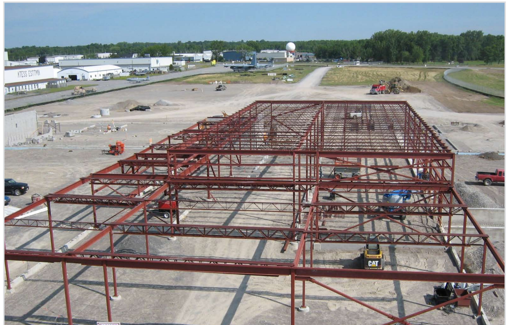
A view of the construction site for a future Joint Nuclear Biological Chemical Defence (JNBCD) facility at 8 Wing Trenton. The photo was taken on July 23, 2007.
