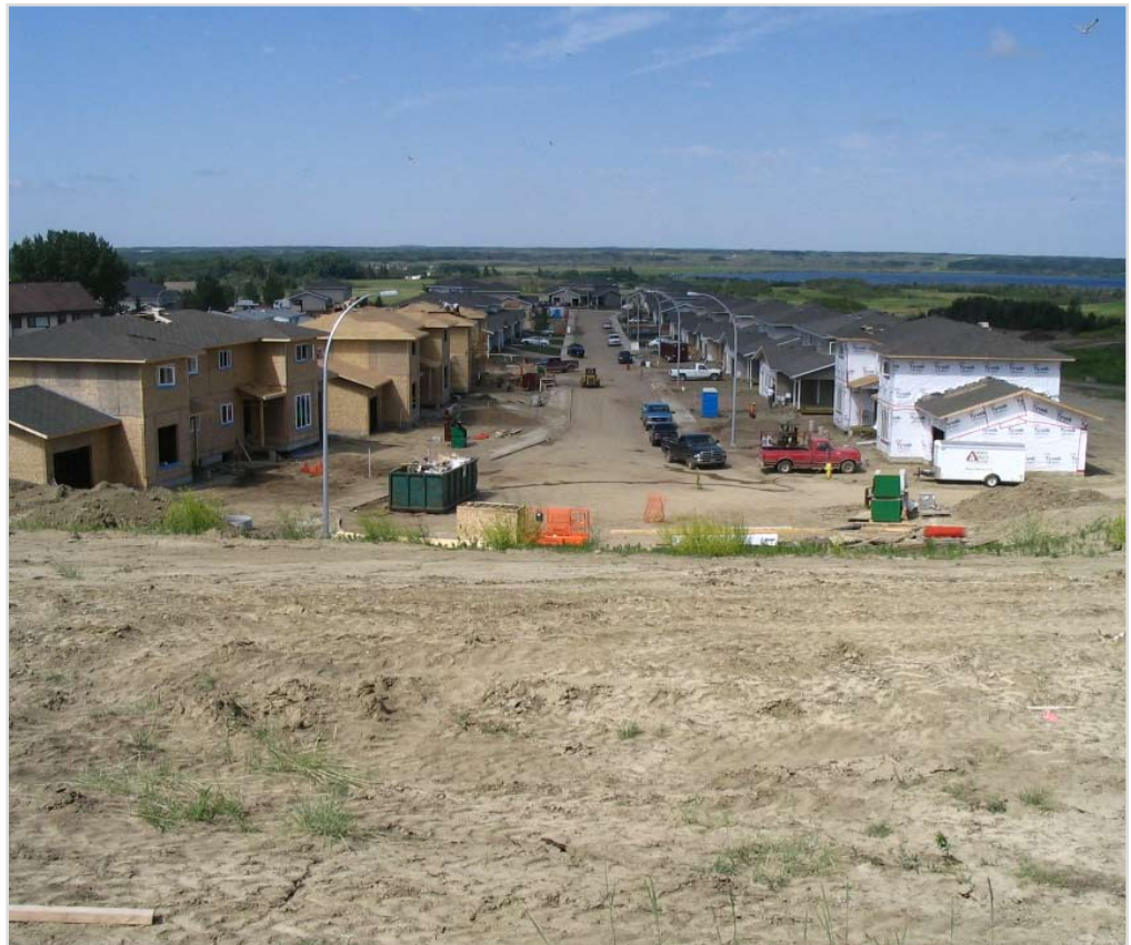
The finishing touches are being put on this $20 million, 60-unit rental housing project at CFB Wainwright.
