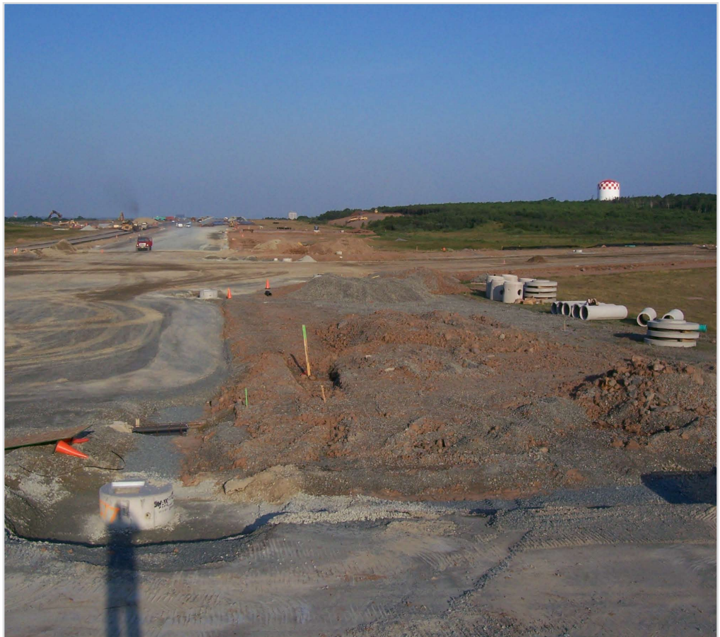
The “first concrete” of the 12 Wing Common Support Facility was poured in mid-July.
