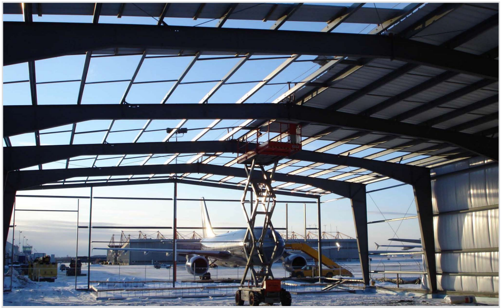
The steel structure of a temporary hangar. The $5.5 million project will be completed on June 18, 2008. The permanent hangar, to be completed in 2010, is currently in the design phase. It is estimated that it will cost more than $90 million to build.
