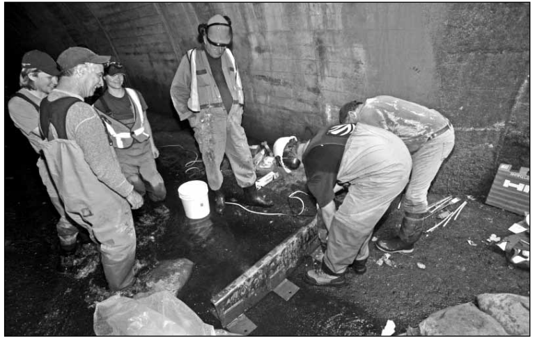
Baffle installation requires the correct ratio of workers to supervisors. Photo: Harry McLeod.
