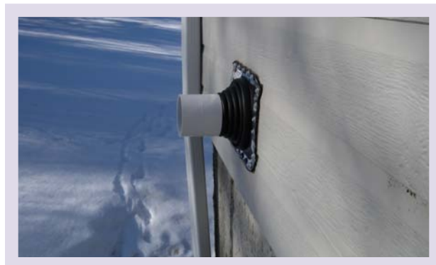
Photo 10 - Example of a ground level exhaust discharge
