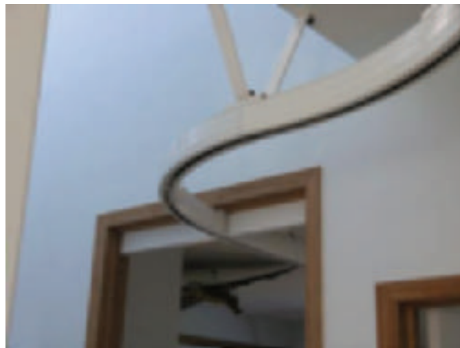
Figure 27 —ID#10 Door jamb
