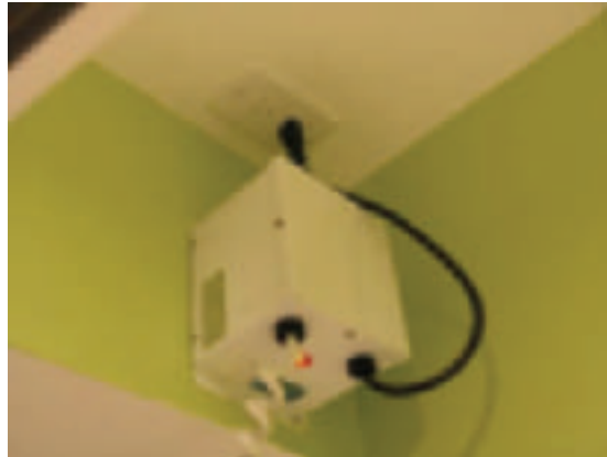
Figure 11 —ID#02 Power supply
