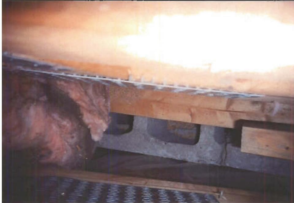
Photo 07: Site 1, Air Leakage Path at Party Wall
