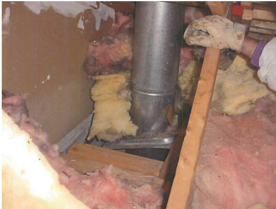
Photo 04: Site 1, Air Leakage Path at Chimney
