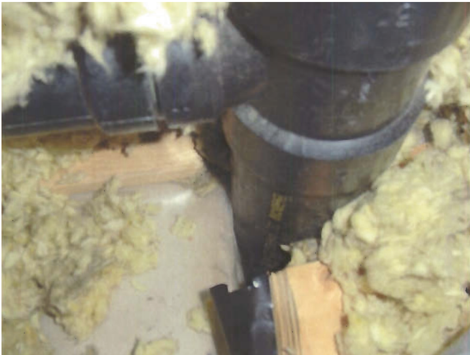
Photo 42: Site 4, Air Leakage Path at Plumbing Vent
