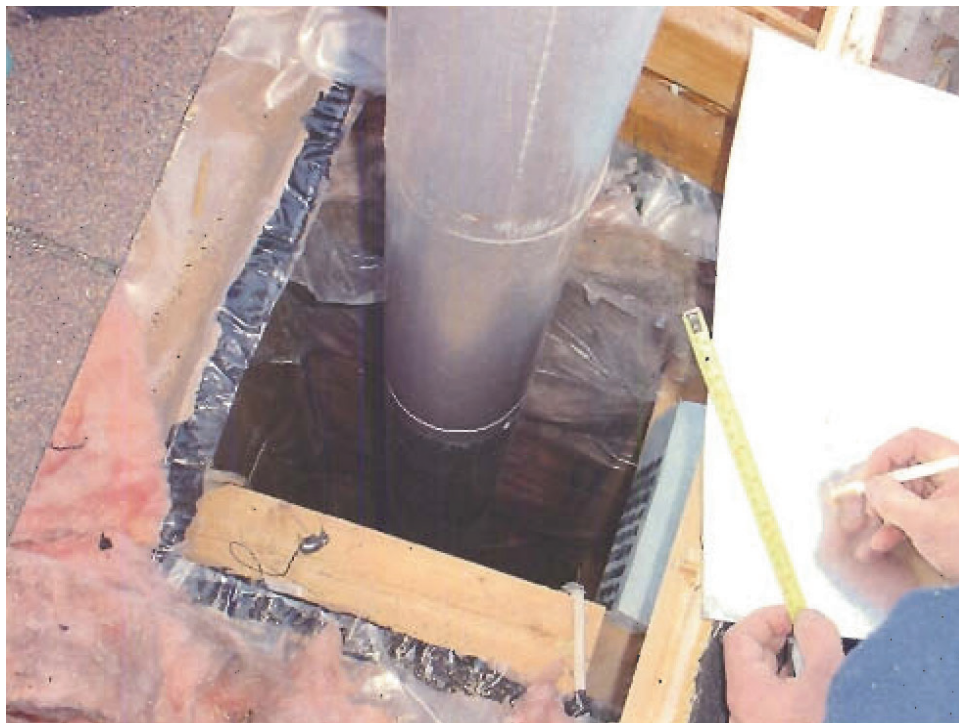
Photo 06: Site 1, Air Leakage Path at B-Vent (Furnace) Chimney
