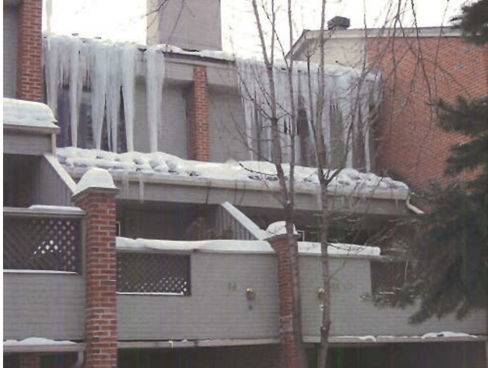
Photo 03: Site 1, Typical ice formation
