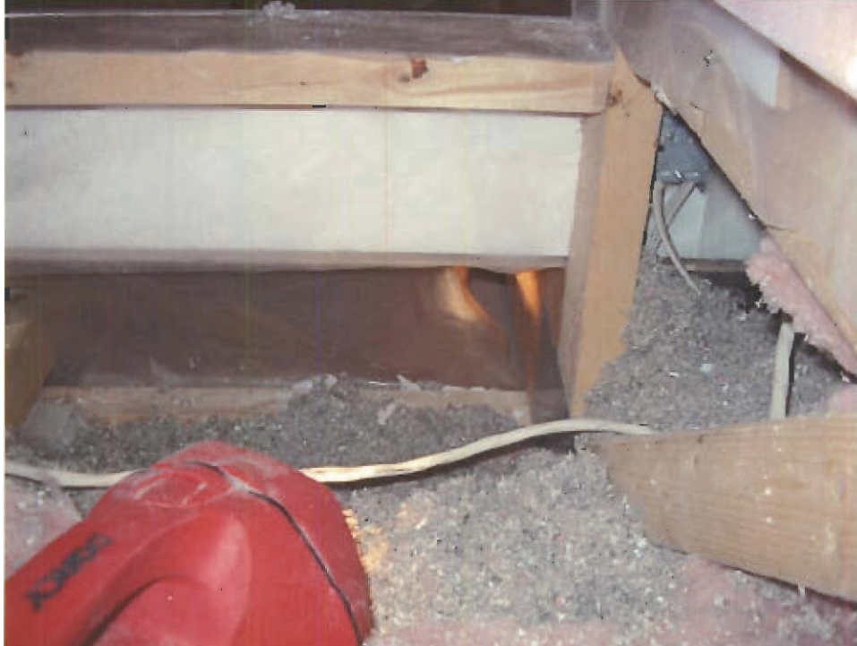
Photo 31: Site 3, Air Leakage Path at Base of Wall
