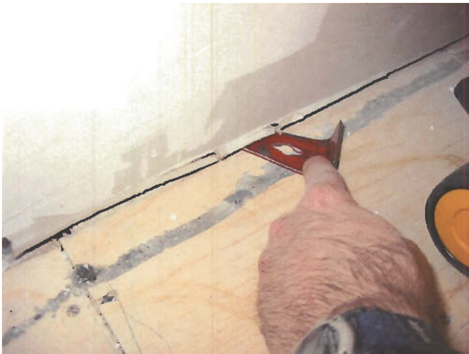
Photo 32: Site 3, Gap at Base of Knee Wall
