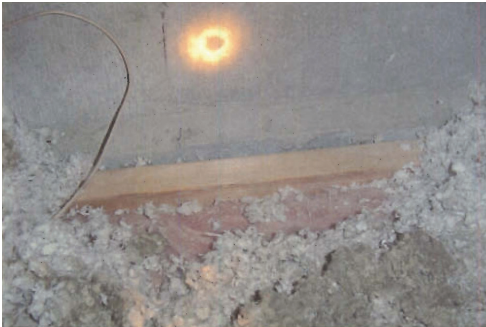
Photo 20: Site 2, Air Leakage Path at Party Wall
