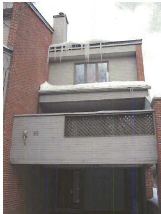
Photo 12: Site 1, Unrepaired Unit, February 19, 2004
