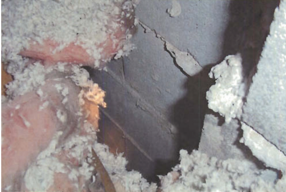
Photo 19: Site 2, Large Air Leakage Path at Party Wall
