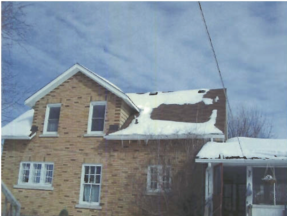
Photo 62: Manotick, Post Repair Snow Cover - Dormer
