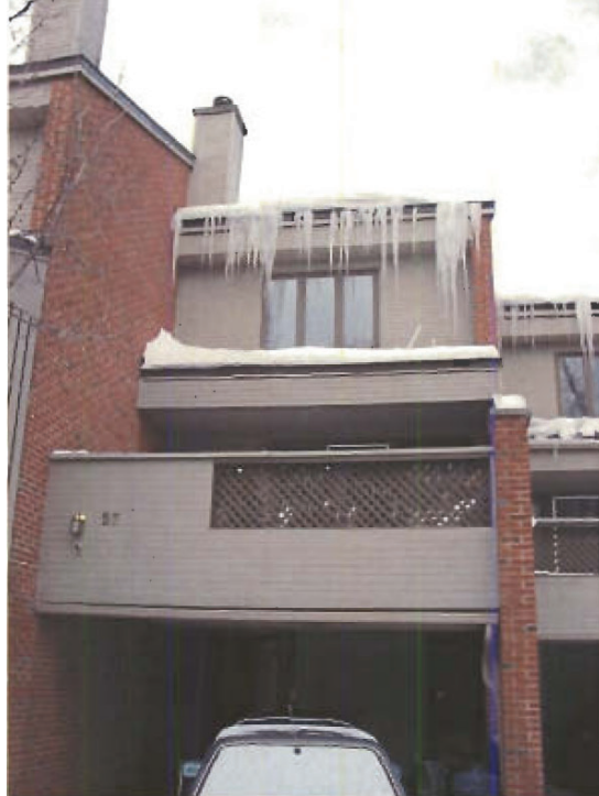
Photo 11: Site 1, Unrepaired Unit, February 19, 2004
