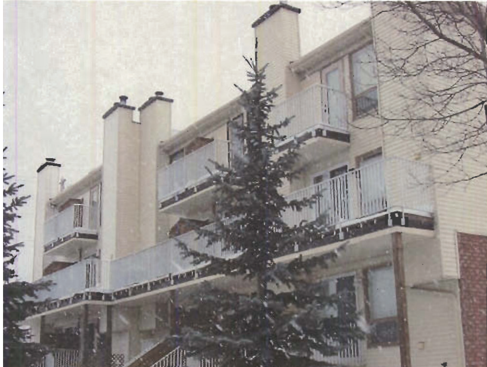
Photo 49: Site 4, Unrepaired Unit Wall (back), January 20, 2004
