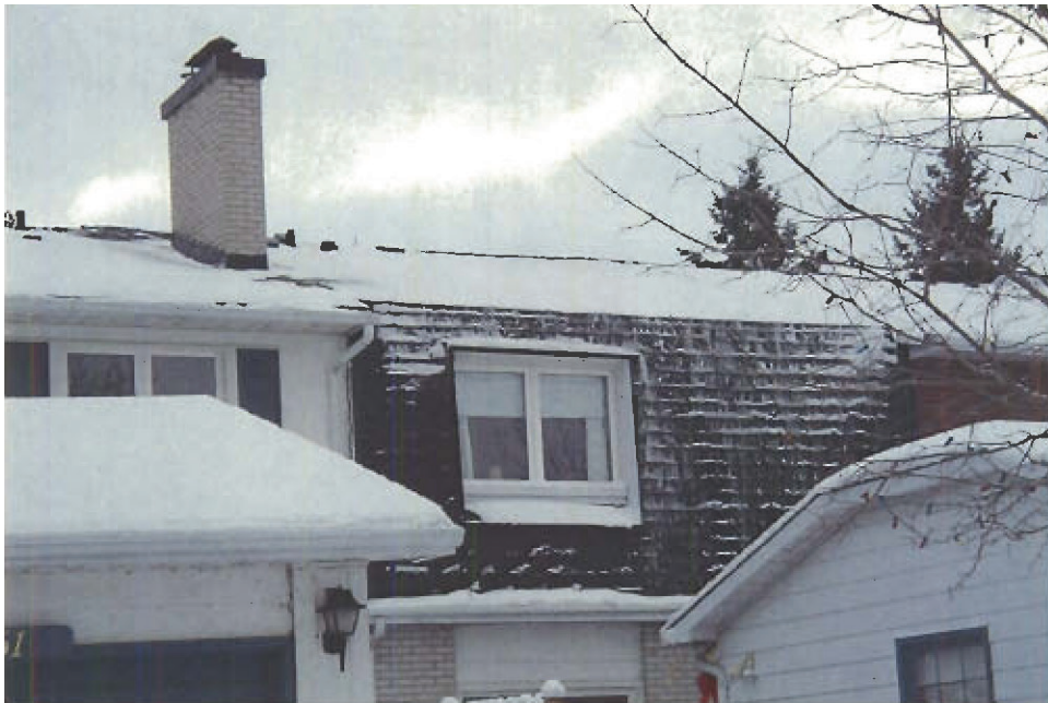
Photo 18: Site 2, Ice Formation on Mansard Style Roofs
