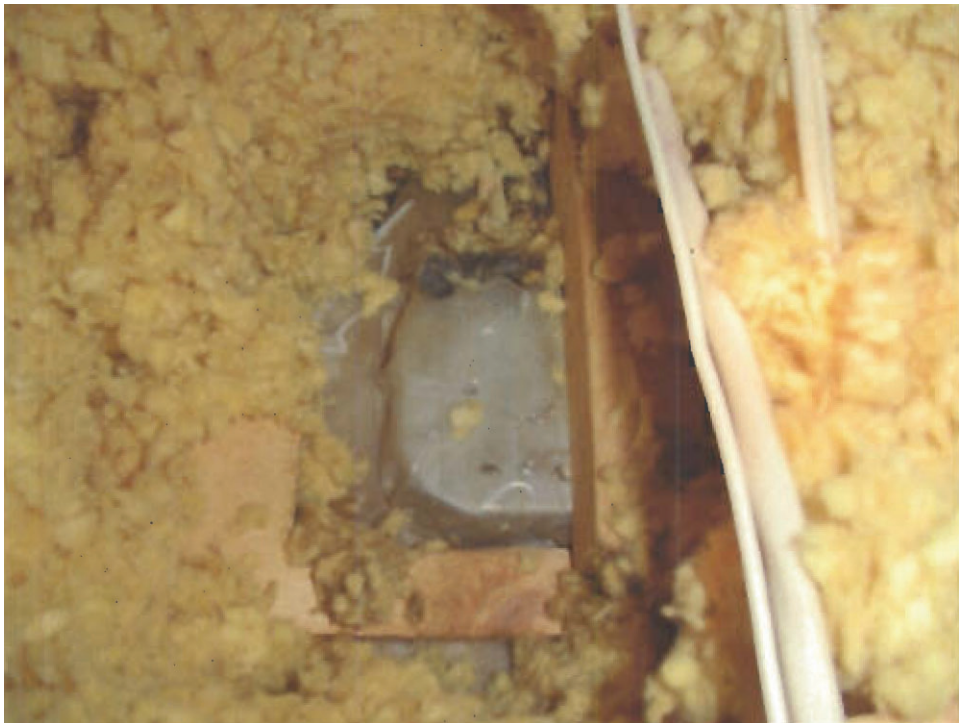
Photo 44: Site 4, Electrical Box in Ceiling
