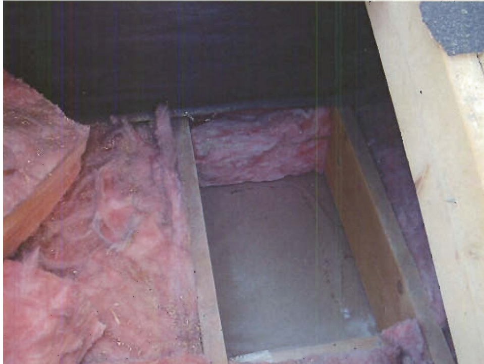
Photo 05: Site 1, Air Leakage Path at Joist Penetration
