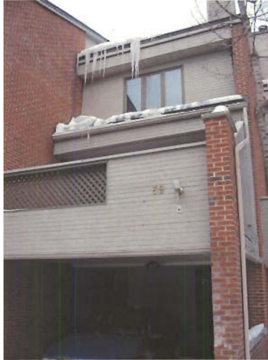
Photo 13: Site 1, Unrepaired Unit, February 19, 2004
