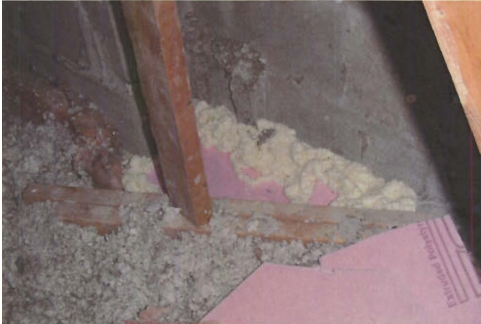
Photo 21: Site 2, Air Sealing Repairs at Large Air Leakage Path at Party Wall
