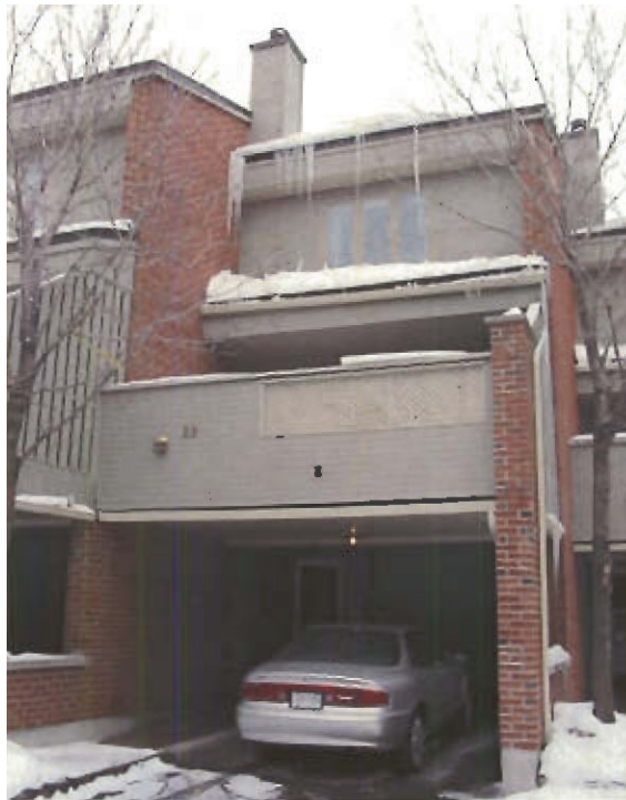
Photo 14: Site 1, Unrepaired Unit, February 19, 2004
