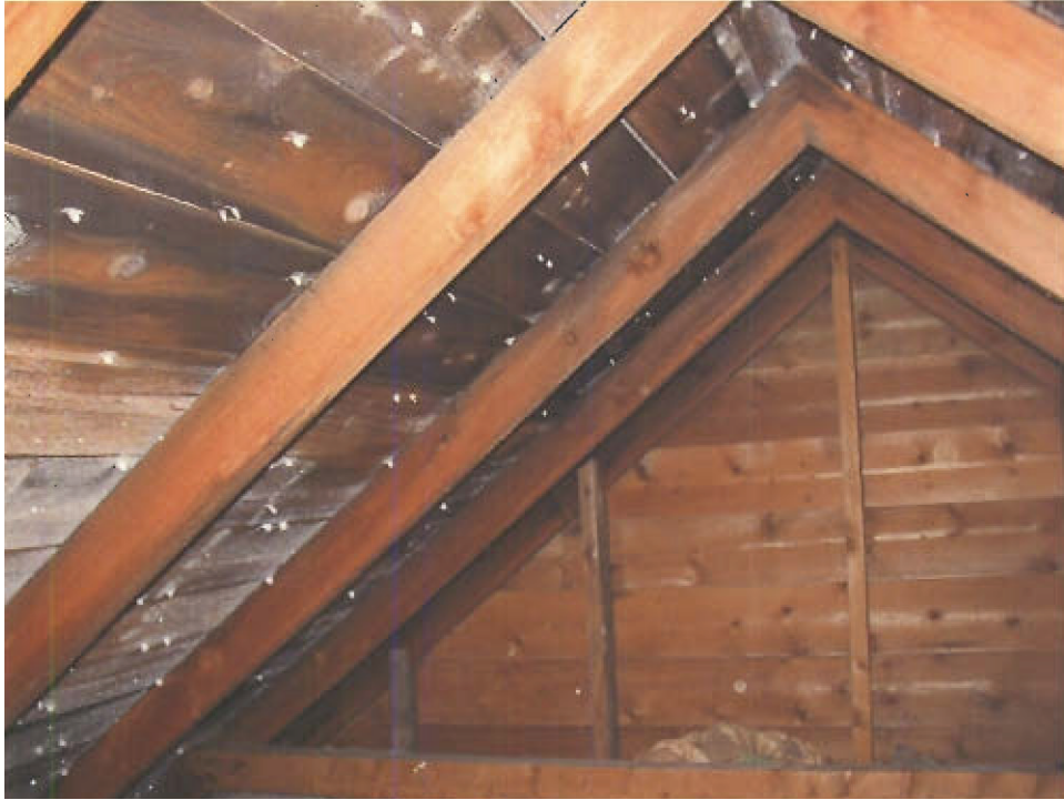
Photo 56: Manotick, Front on Underside of Sheathing
