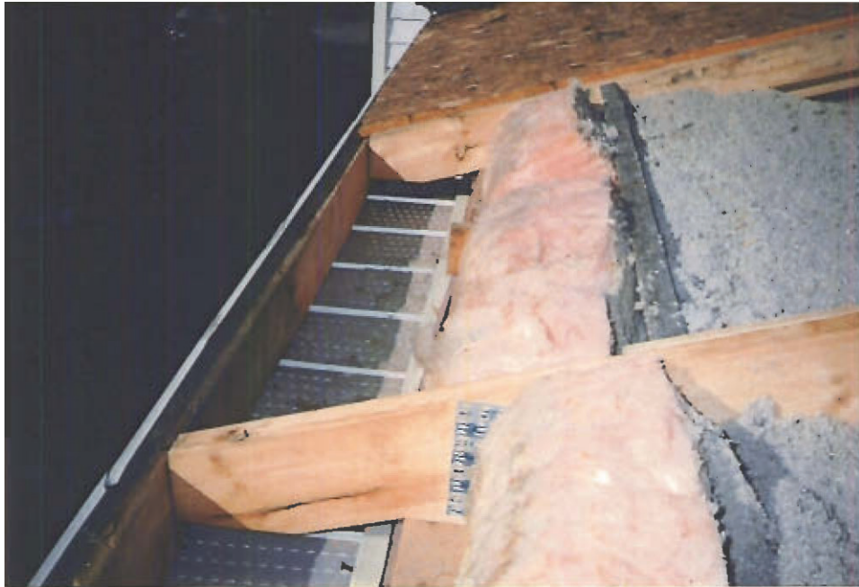
Photo 41: Site 4, Blocked Soffit Ventilation
