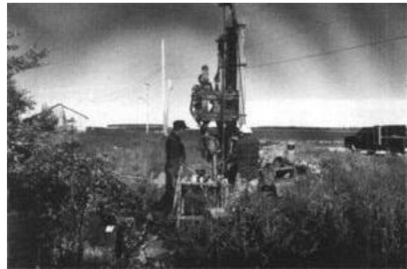
Drilling carried out during the environmental characterization of a site in Eastmain in 1997.
