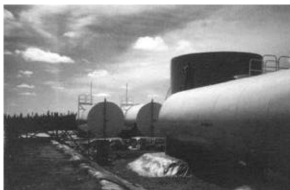
Tanks being installed in 1997 to increase the fuel storage capacity of the Waskaganish electric power station.
