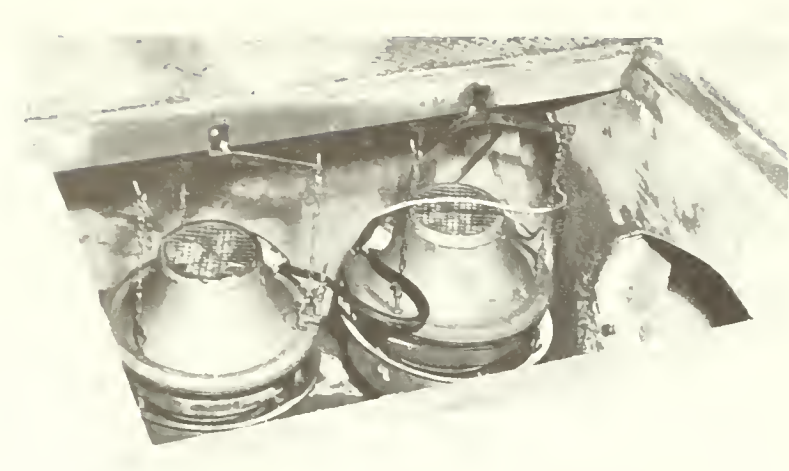
Fig. 28 Centrifugal humidifier installed in supply duct.
