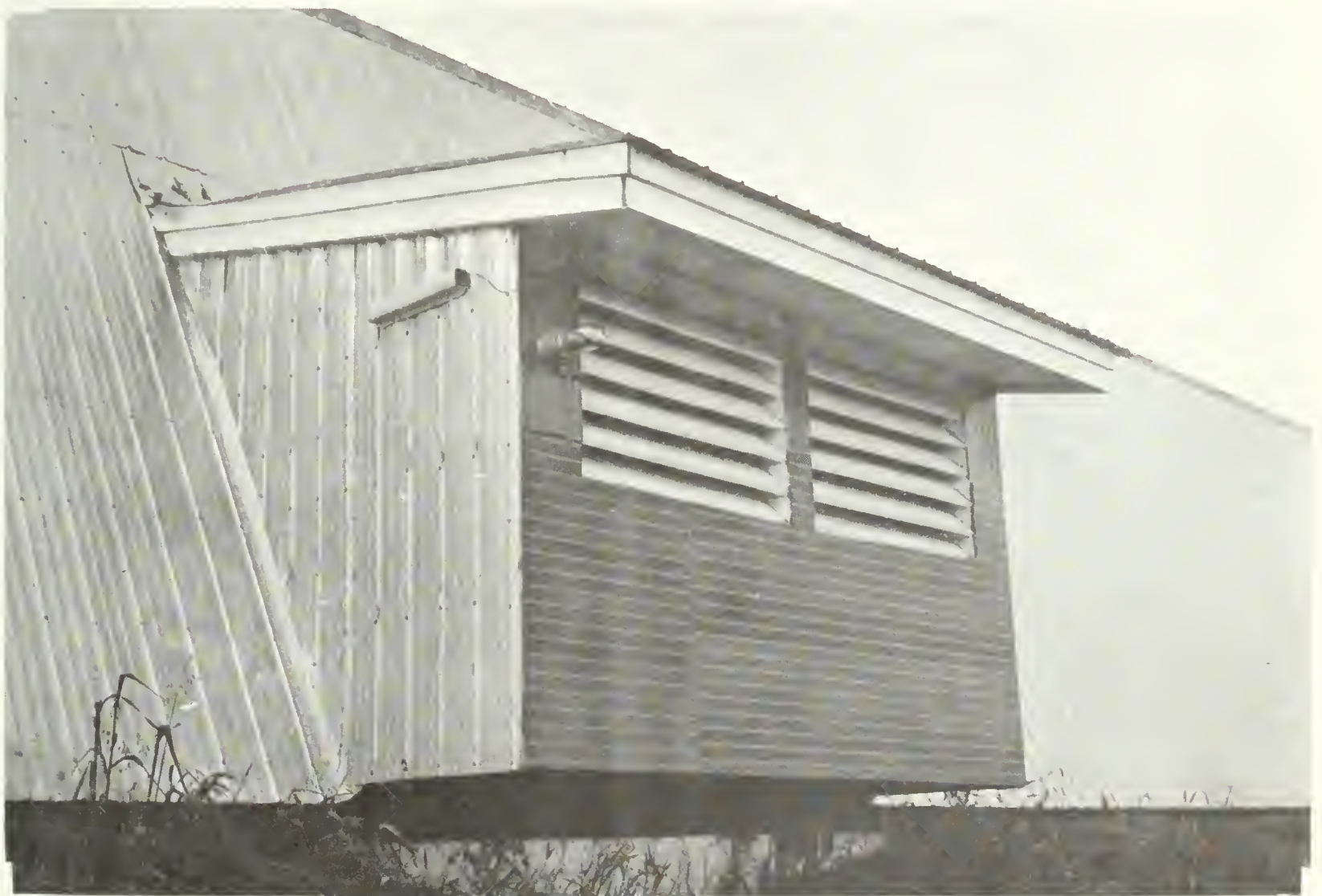
Fig. 19 Air intake and exhaust housing showing exterior bulb of differential thermostat and system failure warning light.
