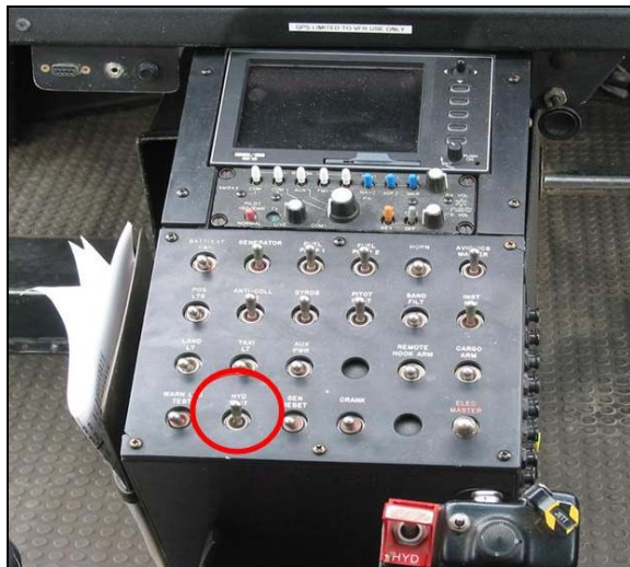
Photo 2. Hydraulic accumulator test switch
