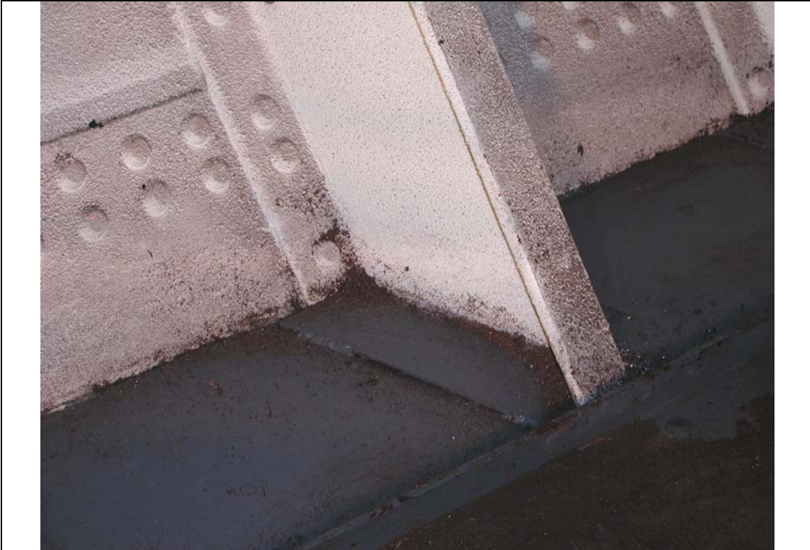
Figure 5.2C. Broom clean in way of stiffeners. Remaining material is loose oil absorbent material.
