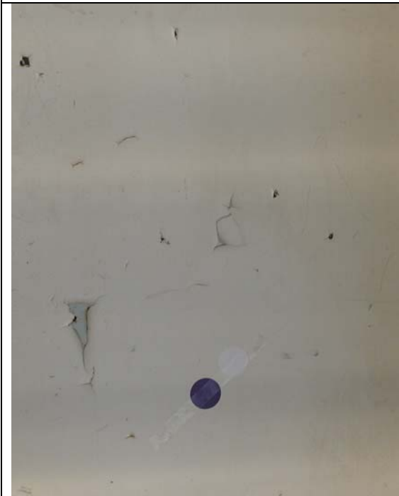
Figure 7.2C. Small chips of loose and flaking paint. Black/ white dots are 4cm diameter.
