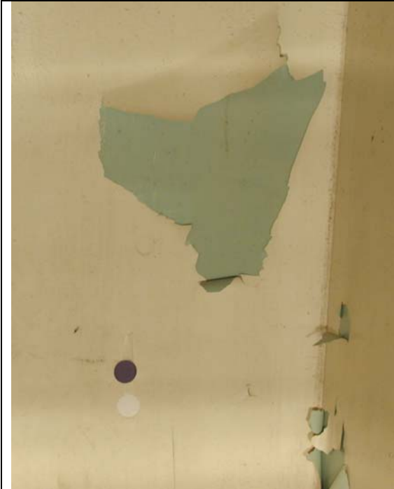
Figure 7.2A. Large chips of loose and flaking paint. Black/ white dots are 4cm diameter.
