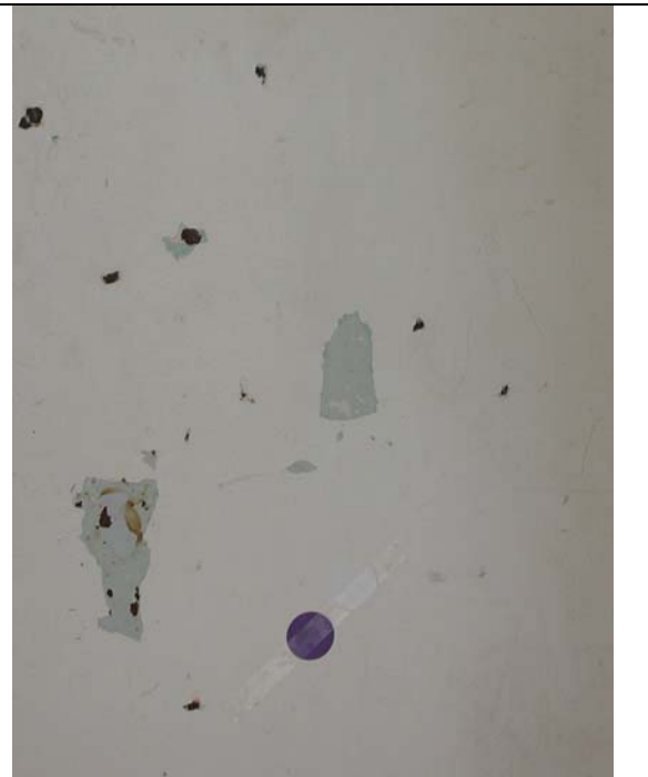
Figure 7.2D. Loose and flaking paint – required degree of removal.
