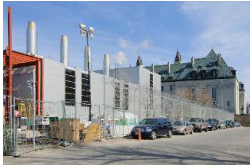
Cliff Central Heating and Cooling Plant—1 Fleet Street, Ottawa, Ontario, street view, Crown-owned
