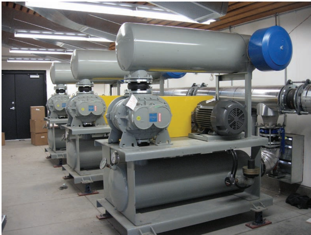
Lagoon Aeration Blowers
