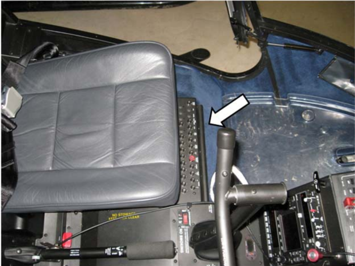
Photo 4. Left breaker panel
