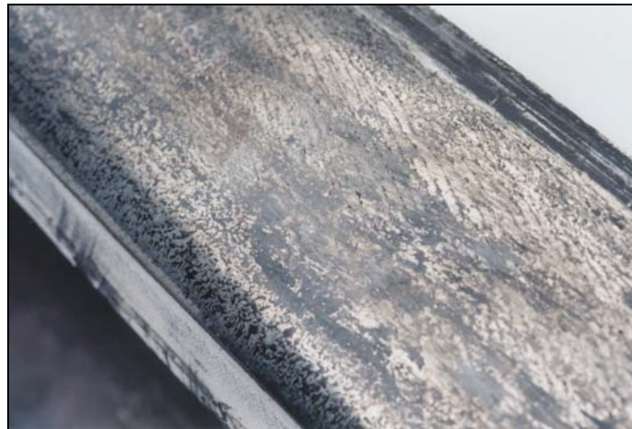
Photo 5. Head checks in larger piece of recovered rail
