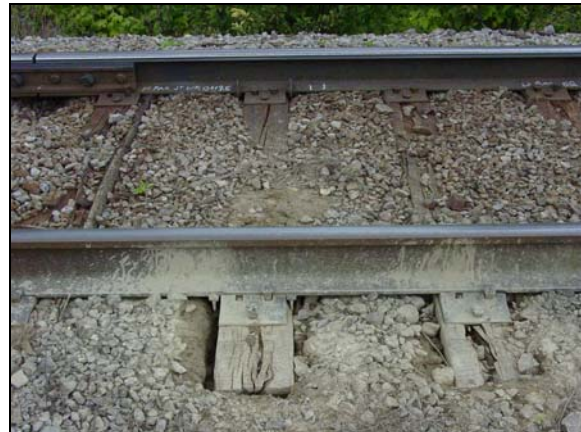
Photo 2. View of tie conditions on low rail of six-degree curve
