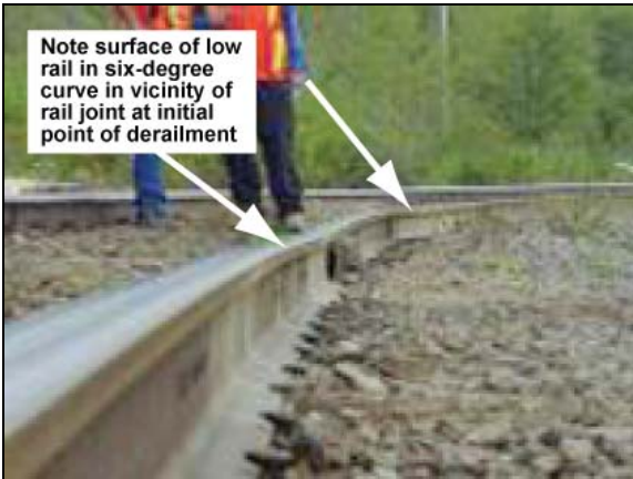
Photo 1. View of track surface looking northward from low rail in six-degree curve
