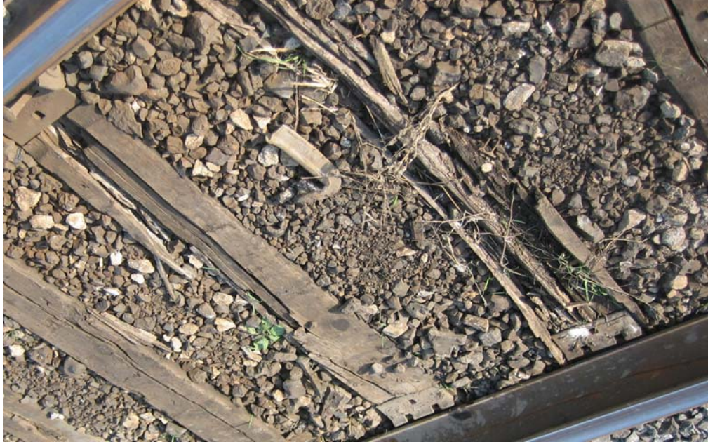
Photo 3. Tie condition in the vicinity of the derailment
