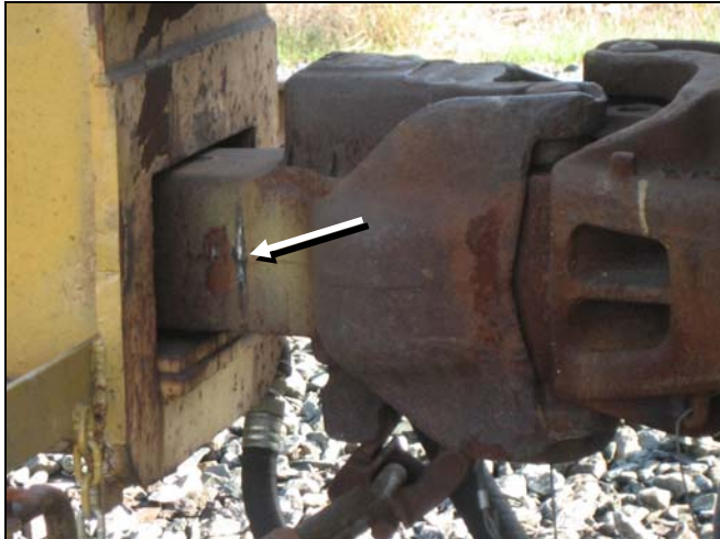
Photo 2a. Severe gouging on the side of the coupler shank of car BGSX 122226
