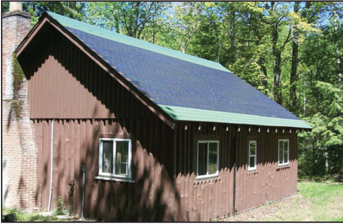
Sullivan's Cabin with Photovoltaic Collector Shingles at Pictured Rocks National Lakeshore Photograph courtesy of Gregg Bruff, National Park Service
