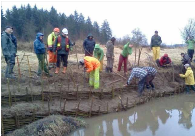
Bioengineering workshop participants build a wattle fence along Silverdale Creek. Photo: Natashia Cox
