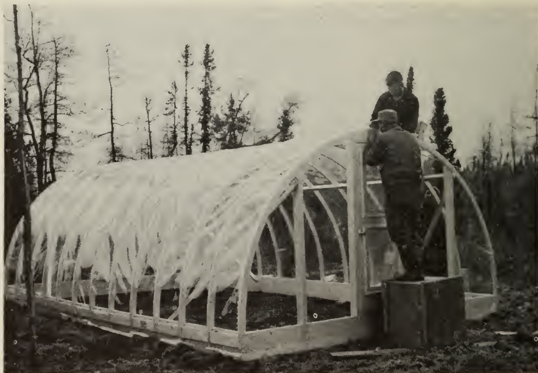
Figure 11 – Greenhouse with laminated plywood rafters at the Experimental Sub-station, Fort Chimo, Que.
