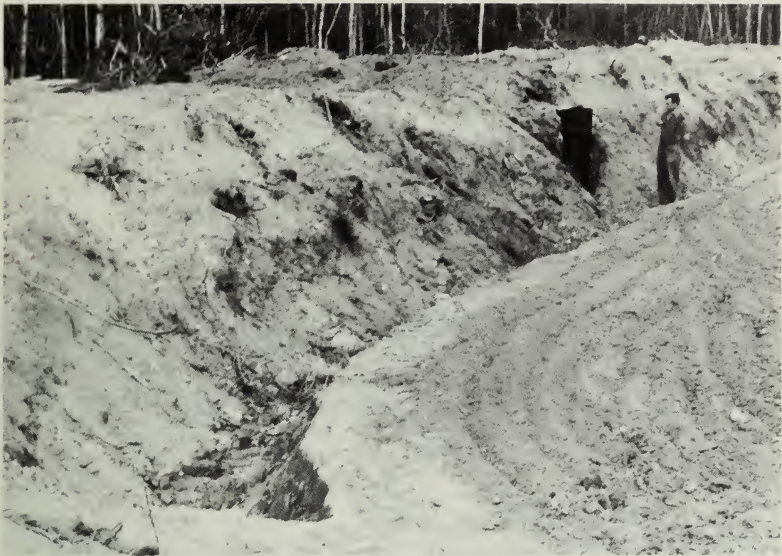
FIGURE 5 The debris from the bog has been pushed into a dyke, the top of which serves as a service road. The ditch around the edge of the dyke drains water into the bulkhead.
